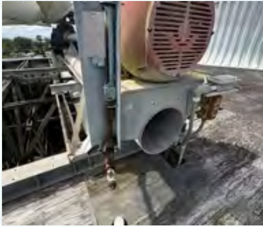
Sample Unit 16 North Gearbox
