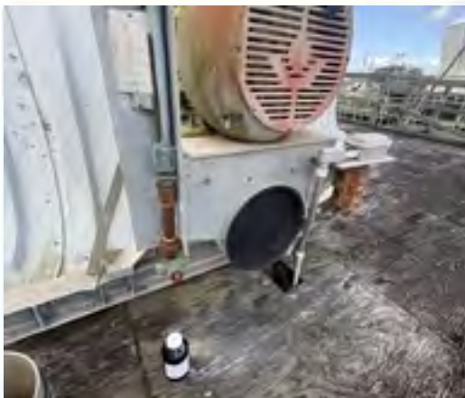
Sample Unit 16 South Gearbox
