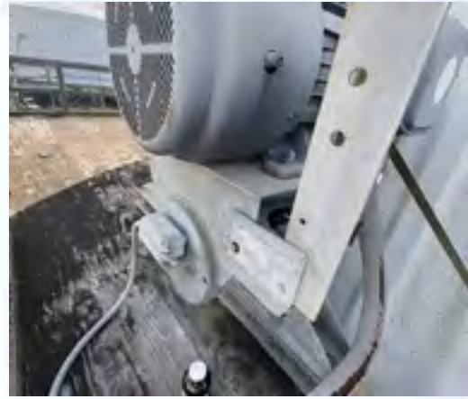
Sample Unit 15 North Gearbox
